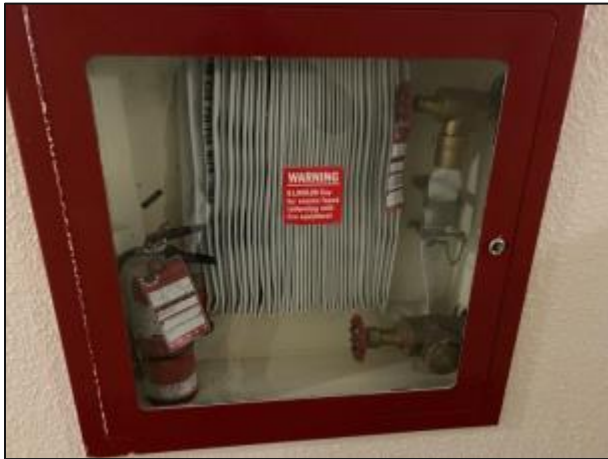
Standpipe Hose & Portable Fire Extinguisher
