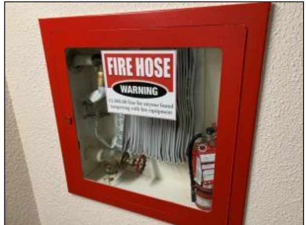
Typical Fire Hose & Extinguisher
