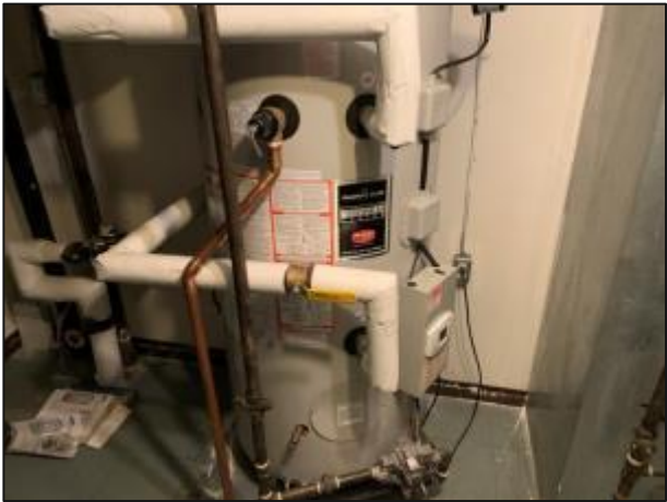
Hot Water Tank
