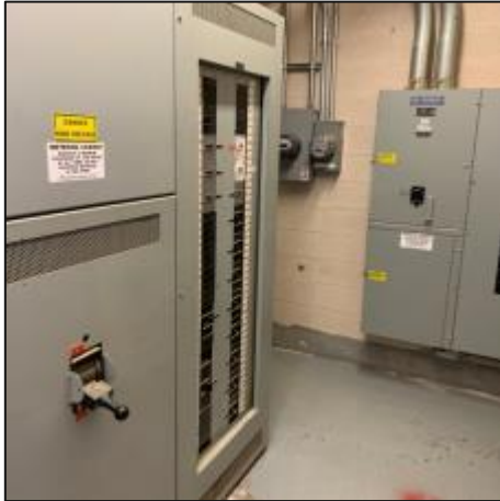
Main Electrical Room
