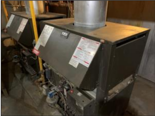
Hot Water Boiler
