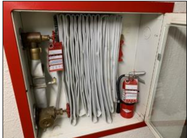
Typical Fire Hose & Extinguisher
