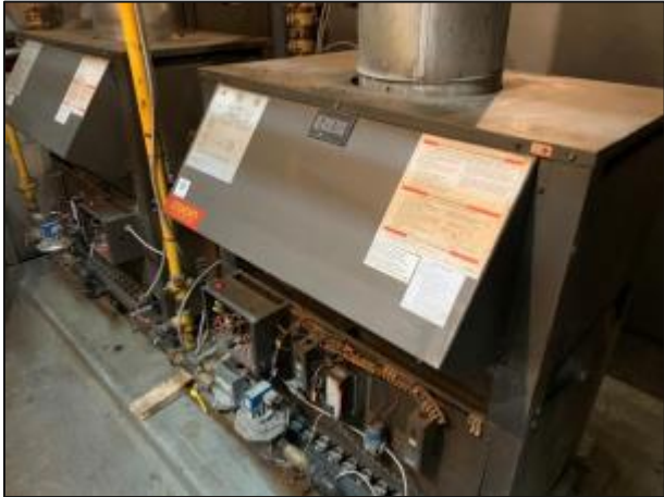
Hot Water Boiler
